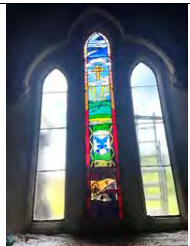
Figure 7 The middle light (Ch.2) is installed. The ladder is positioned to carry on with Ch.3.
